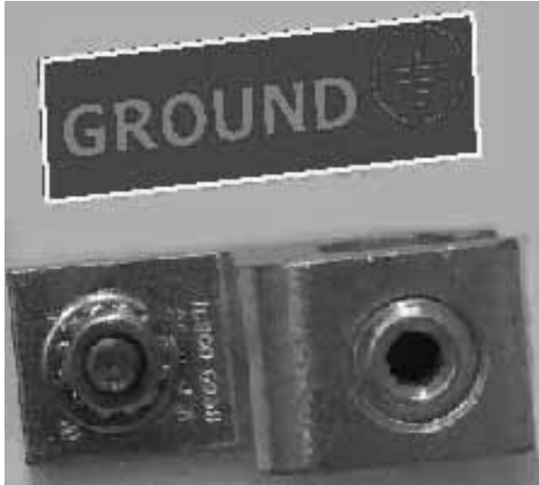
Figure 33. Typical ground stud and label
