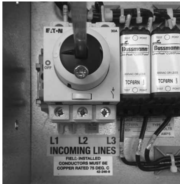
Figure 29. Lower frame incoming lines
